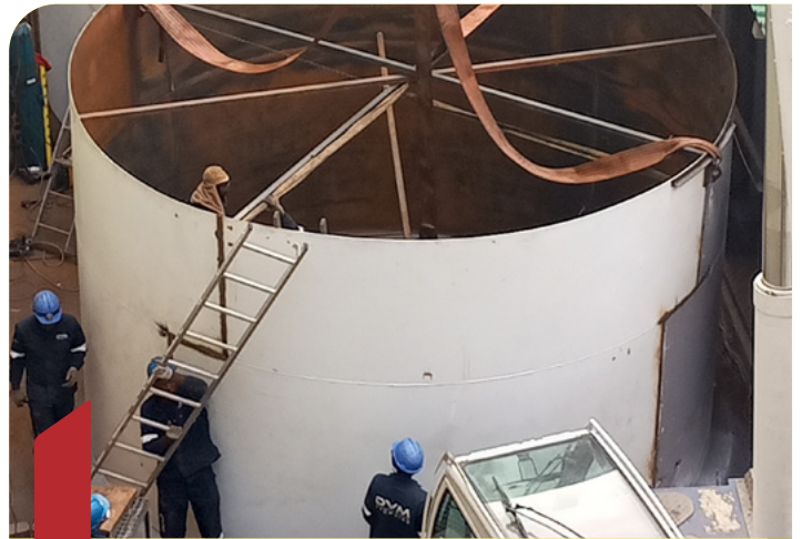
Sulfuric Acid Tank
