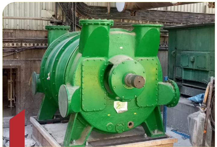
Vacuum Pump installation
